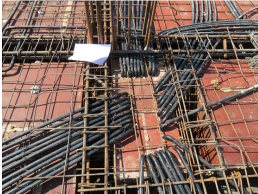
Concealed piping embedded on terrace
