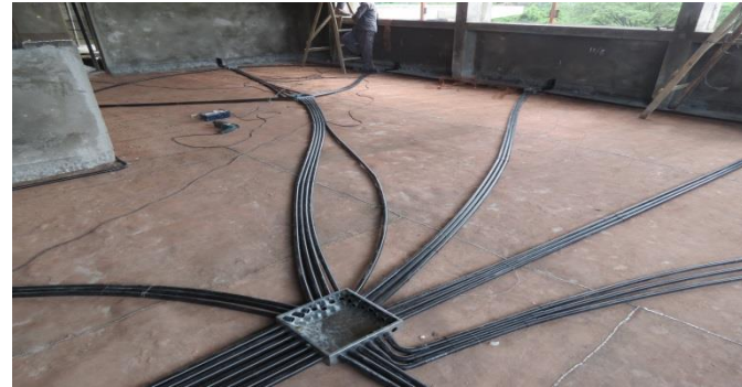
Piping for data & power connection
