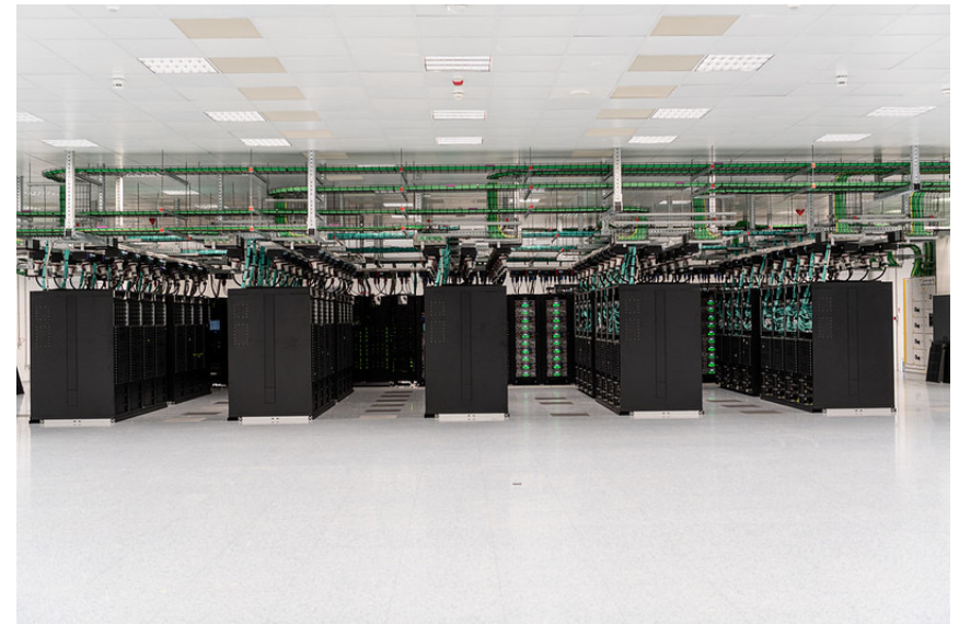
ATOS HPC at Bologna data centre (2022)
